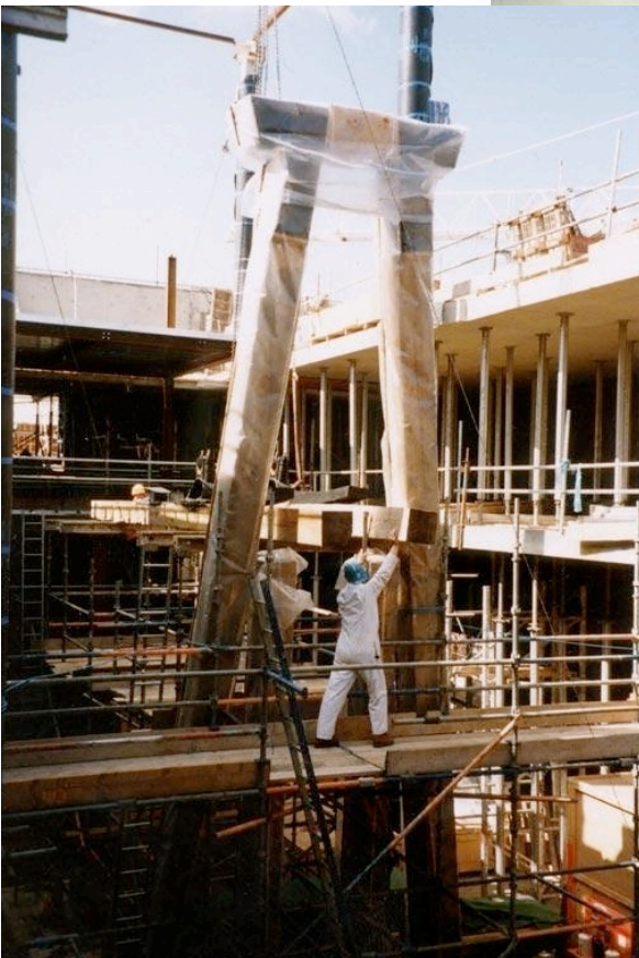
1.13 & 1.14: The Engine being fitted into the Museum of Scotland building site during construction.
